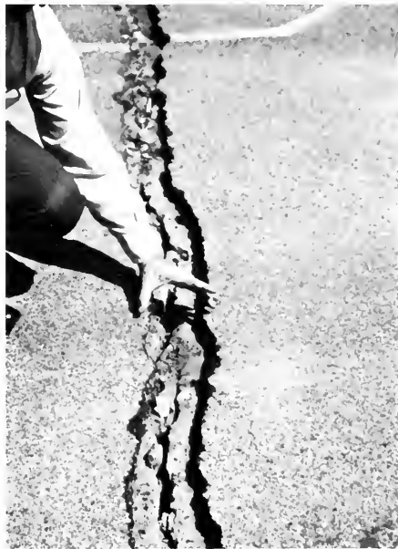
Photo 49. Asphalt paving cracks were almost invariably much wider than the soil cracks.
